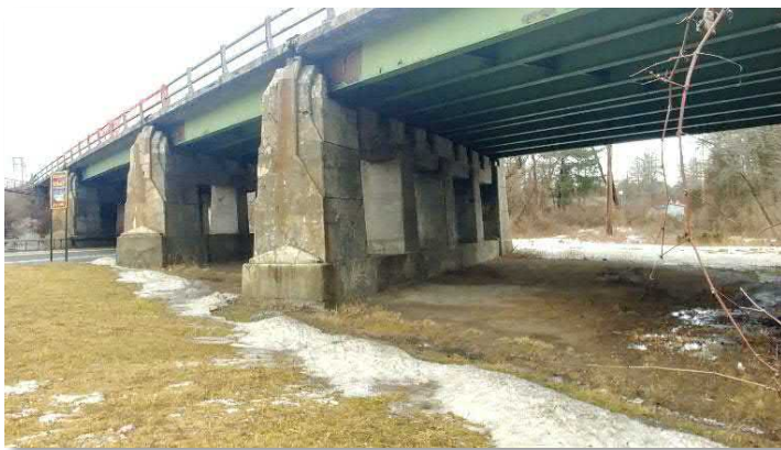
Figure 24 Looking north at the Route 9H bridge. The AHET will pass under the bridge pier opening on the right side of this picture
